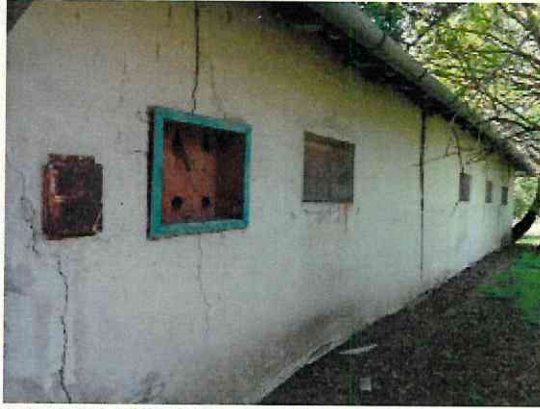
(/kepek/2018/04/21/80682_tessedik_tanya_007_large_normal.jpg) A falakon komoly repedések vannak.
